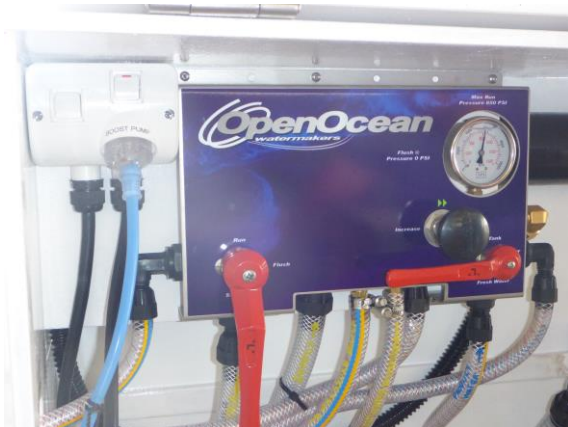
Control Panel and switches
